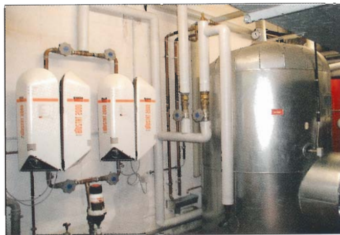
Above. Two BST50 units mounted in parallel. The cold water service is protected by a Judo Profi backwash filter.
